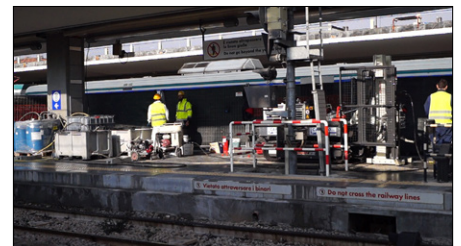
Fig. 6, Injection of PlumeStop on the platform of the railway station, in Area 3;
